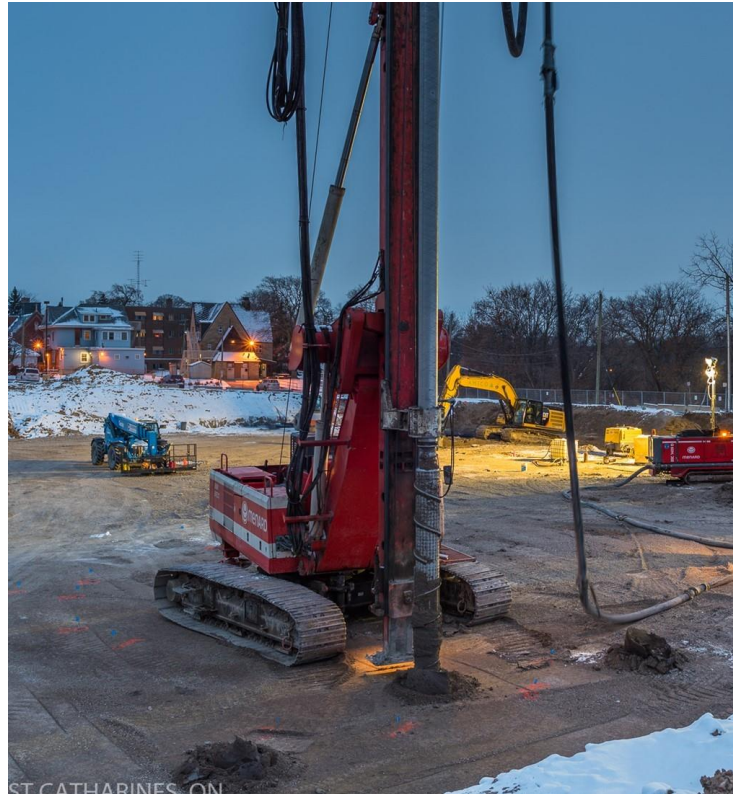
Figure 1: CMC Installation in St. Catharines, ON
